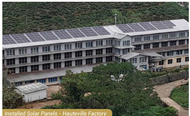
Installed Solar Panels - Hauteville Factory
